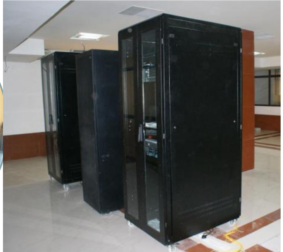
Data Center (Health Knowledge Park)
